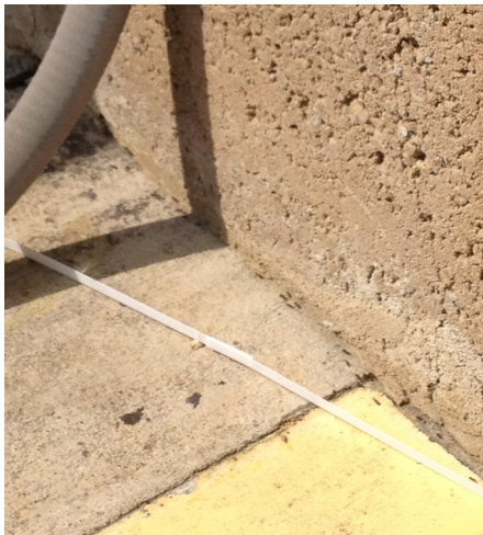
OHA following edge of concrete pad and foundation wall as a guideline between the dumpster and kitchen. Photo: Karen Vail, UT Entomology & Plant Pathology
