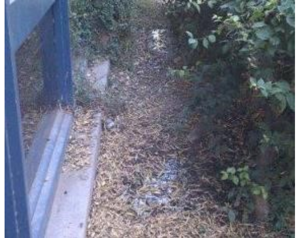
Fig. 6. Fallen leaves and other debris around the building provides harborage for pests and also holds moisture which can weaken the foundation.
