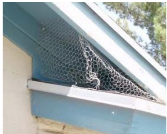
Fig. 7. Wire netting helps to keep birds and rodents out, but needs to be monitored and maintained.
