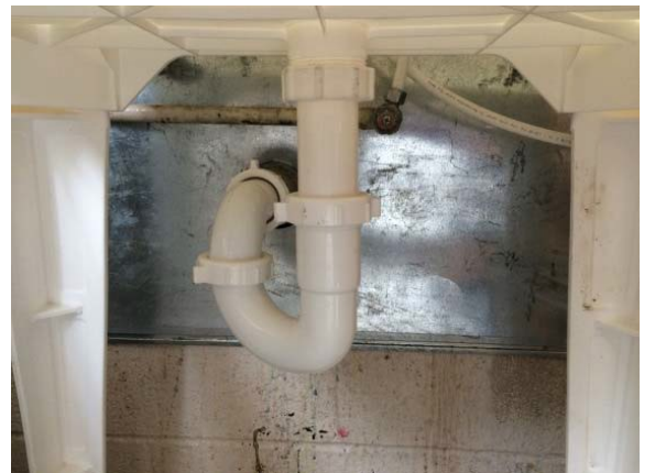
Repair to the opening in the concession stand wall. Pipe penetrations as well as the large gap are well sealed.
