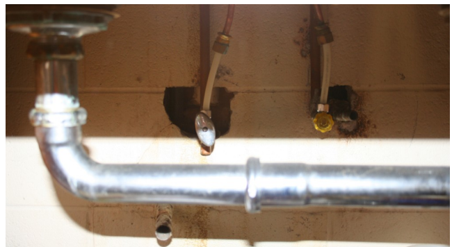
Areas surrounding pipes need to be sealed to prevent mouse entry.
