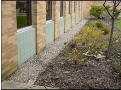
Keep a vegetation-free zone next to a school. Snyder & Gouge, U of AZ.
