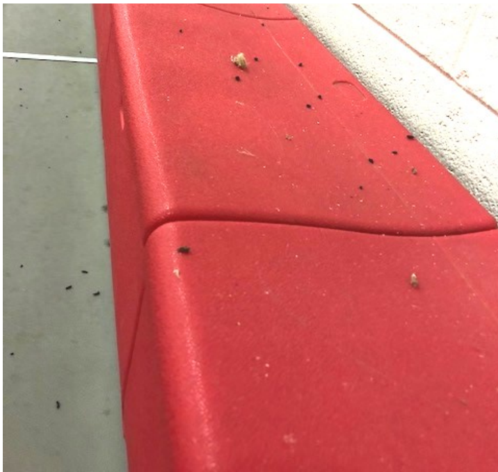
Bat droppings detected during an inspection of a demonstration school.
