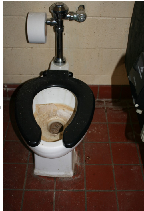
An unused toilet lacking water allows American cockroaches easy access to the school.
