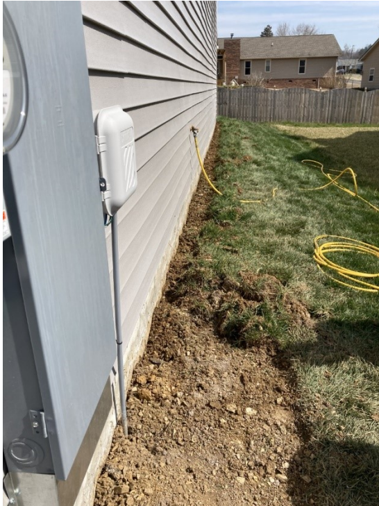
Figure 3. Lush grass being removed 2 ft. from the foundation. Credit: email submission.
