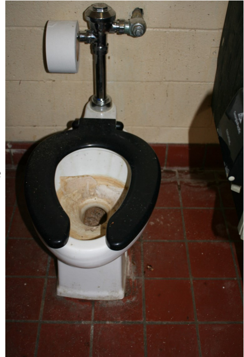
An unused toilet lacking water allows American cockroaches easy access to the school.
