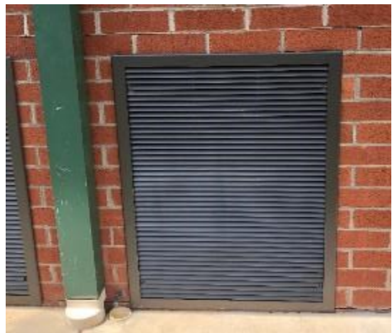
Figure 19. Each exterior room has a vent that would be difficult to screen, allow air flow and keep millipedes out.
