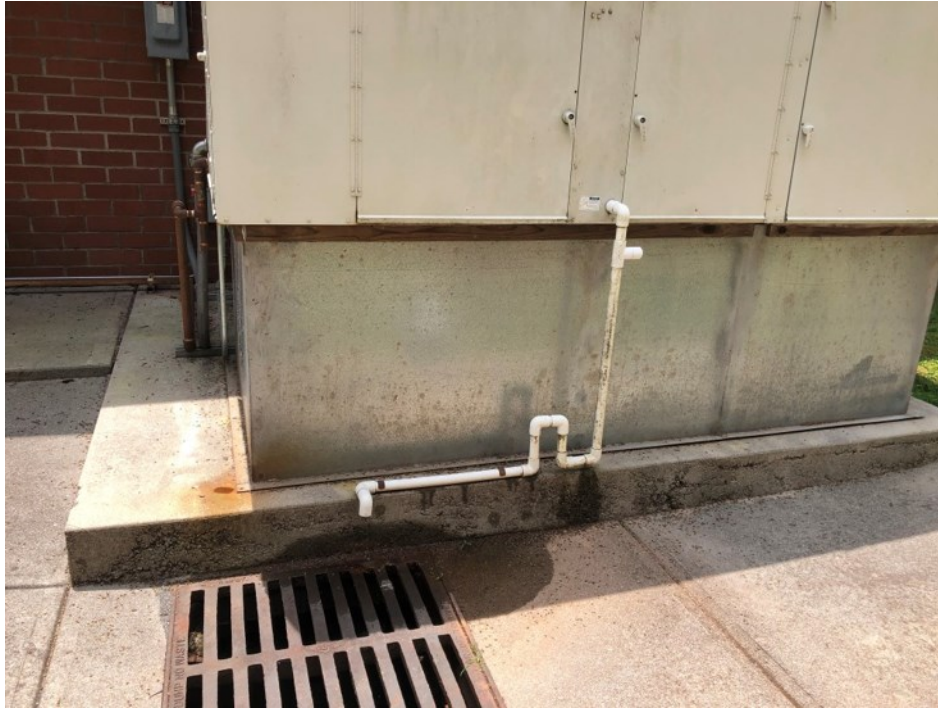
Figure 7. Condensation from the AC unit is led to the drain.
