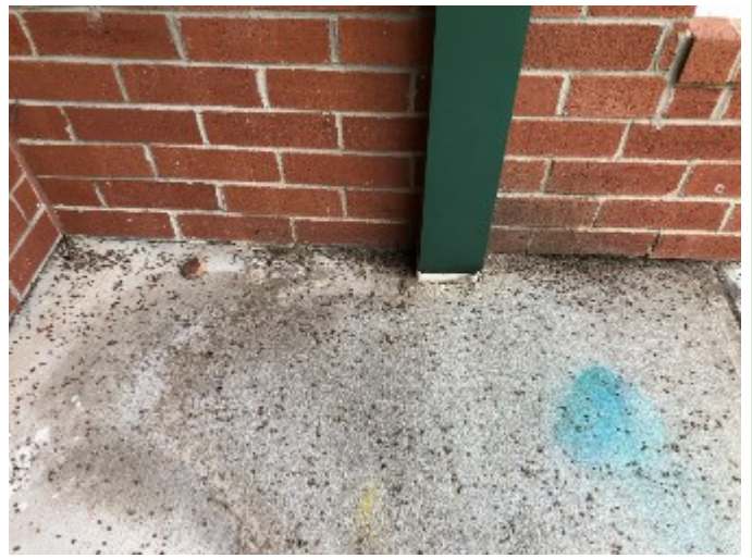
Figure 6. A tremendous number of millipedes were found in this corner close to the downspout.
