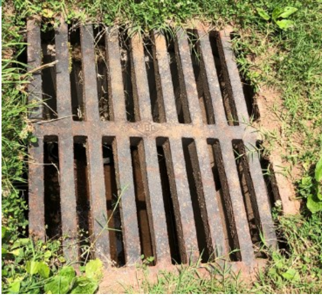
Figure 9. The drainage system runs through the grass on the north side of the school and before the red shale bank.
