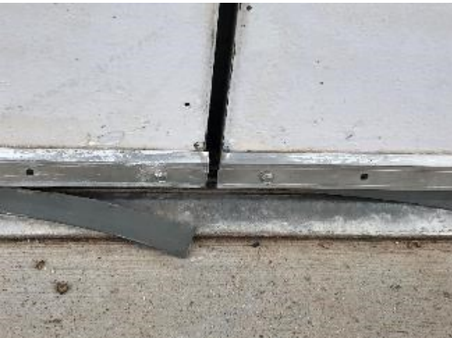
Figure 18. Damaged door sweeps and gaps between doors. Brush sweeps and astragal (brush between the doors) would seal the doors better.
