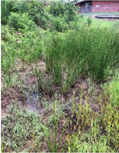
Figure 13. A small wet area on the northwest corner of the school.
