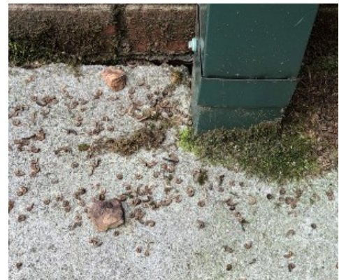
Figure 12. Millipedes were abundant at the base of this downspout too.
