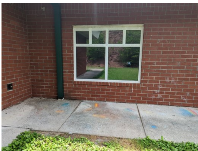
Figure 5. Chalk art drew us to this section, but it wasn't the main attraction.
