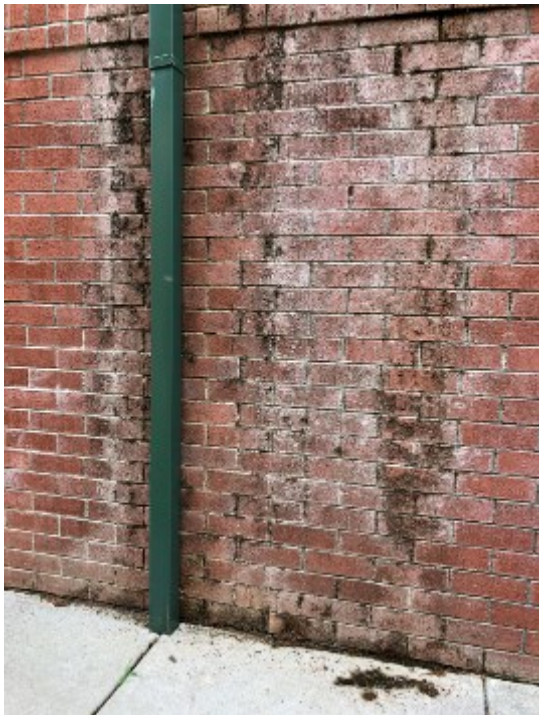
Figure 11. Moss growing on the exterior of the building was probably due to a prior drainage system or damaged roof.
